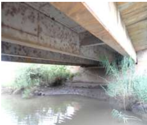
Figure 4.2: Corrosion Defect due to Reinforced Rust within the Concrete
