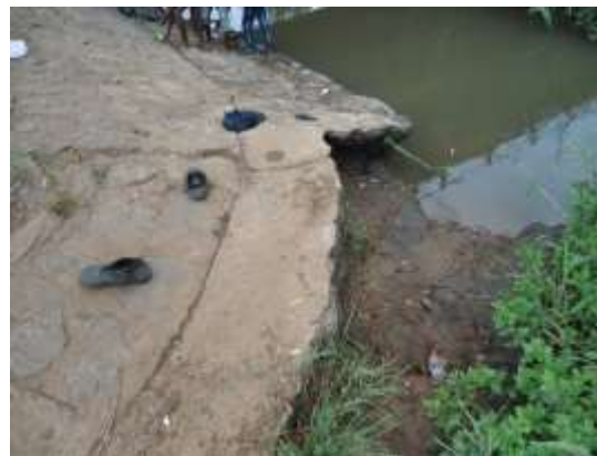
Figure 4.3: Erosion of the Bridge Bank
