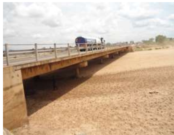
Figure 4.7: Magole VII Side view Scour Depth Defect
