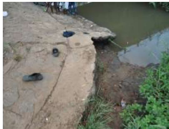
Figure 4.3: Erosion of the Bridge Bank
