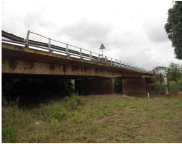
Figure 4.4 Corrosion Defect due to Reinforced Rust within the Concrete
