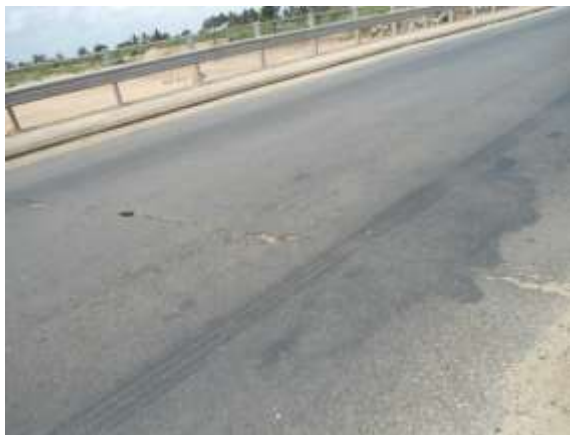
Figure 4.6: Slab Crack Defect
