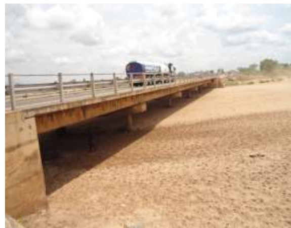
Figure 4.7: Magole VII Side view Scour Depth Defect
